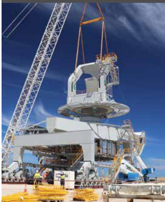
Port Kembla Coal Terminal - Stacker's and Reclaimer
